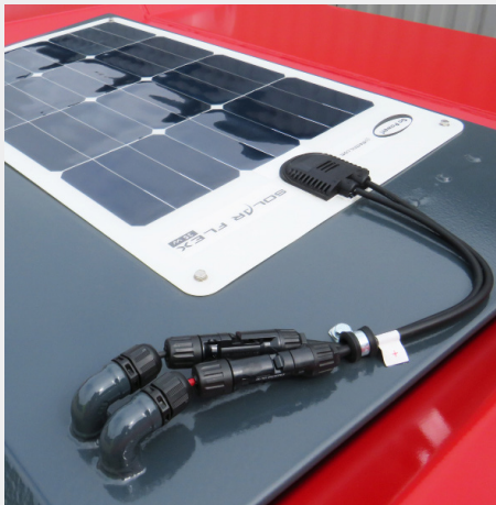
LID-MOUNTED SOLAR PANEL CHARGES FUEL PUMP BATTERY FOR SELF-POWERED DIESEL DISPENSING
